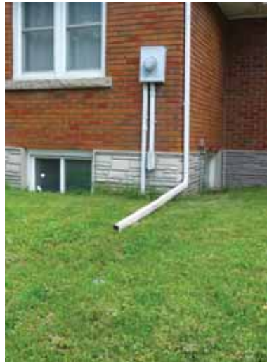
Disconnected downspout Kerry Royer, photographer
