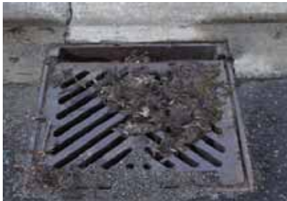
Typical storm drain
