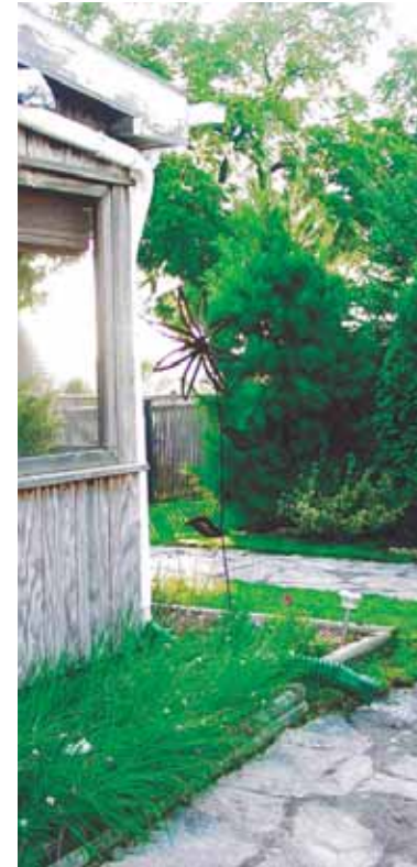
Disconnected downspout Jocelyn Baker, photographer
