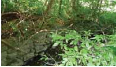
Hardened creek edges
