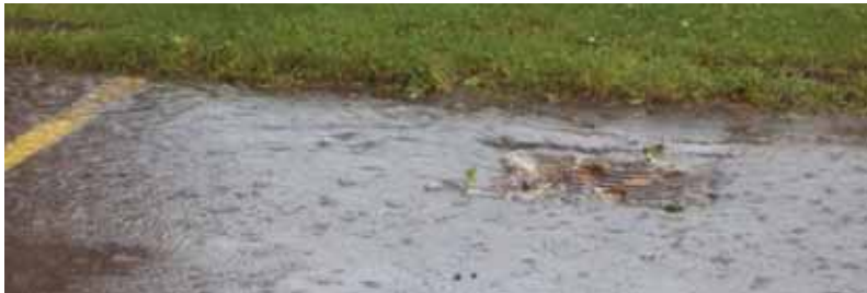
Flooding of storm drain Kelly Jamieson, photographer
