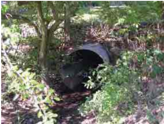
Zone 3 – undersized culvert
